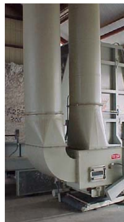
A Hot Box II installed with a fixed head module feeder. Seed cotton travels into the gin with hot air – rocks and green bolls are dropped.
