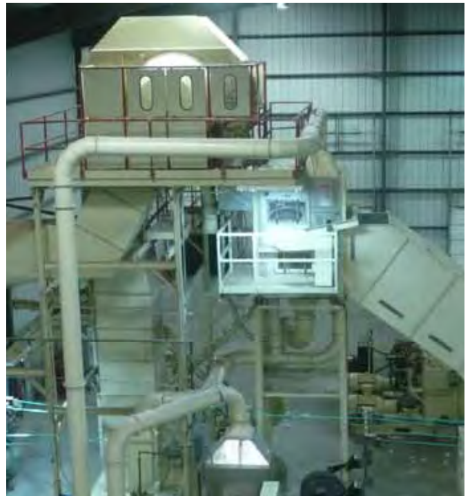
A Steamroller II Lint Conditioning System
