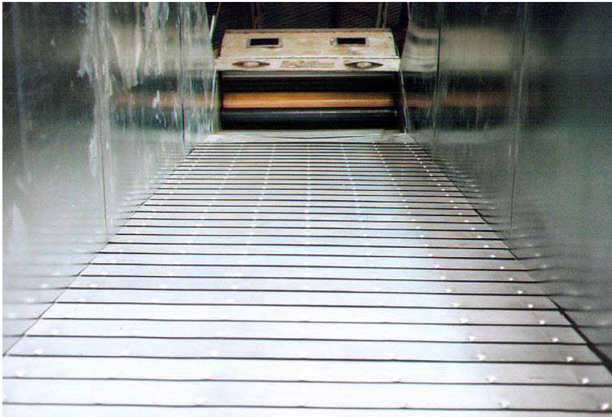
This picture shows a typical Lint Slide Grid installation. It is taken from inside the lint slide looking up at the battery condenser.
